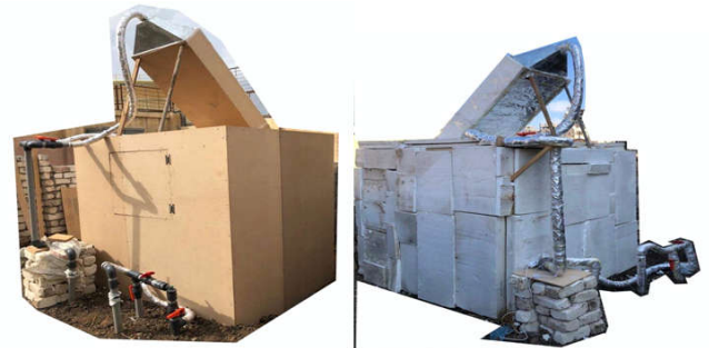
Fig. 4. (a) Room and solar chimney during construction step & (b) Closed-loop experimental system running and in use
