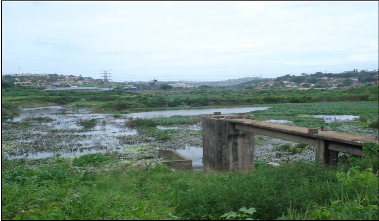
Fig.7. The Diversion Works System (2010) showing the large concrete structure which houses the sluice gates that allows pooled water to flow into the PCS
