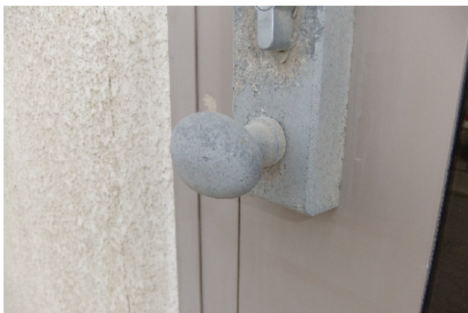
Picture 1. Cast door handle showing extensive top surface corrosion
