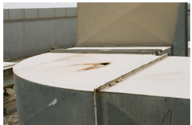
Picture 4. Galvanised steel HVAC duct showing corrosion failure after 3 year's exposure
