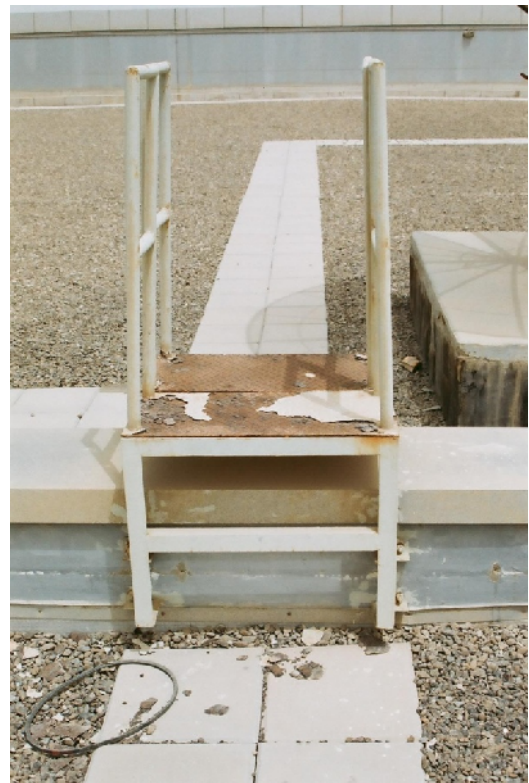
Picture 2. A rarely used walkway. Total coating failure. Age of structure: 3 years
