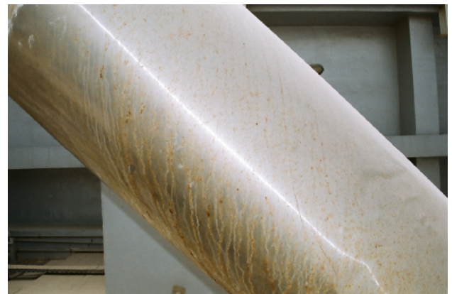
Picture 3. 316L SS HVAC duct showing salt rime and pitting. Two years old
